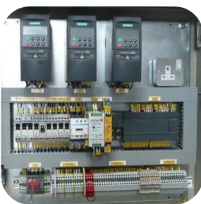
VFD Control Panel
